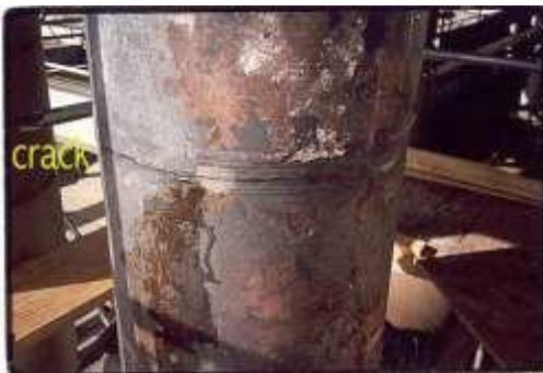
crack Main steam pipe weld failure
