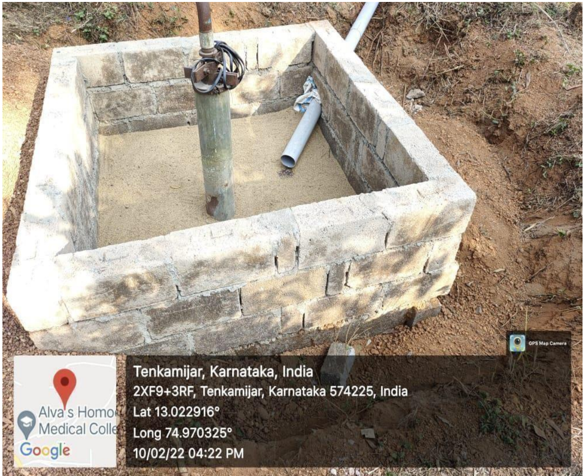
Bore well Recharge pit
